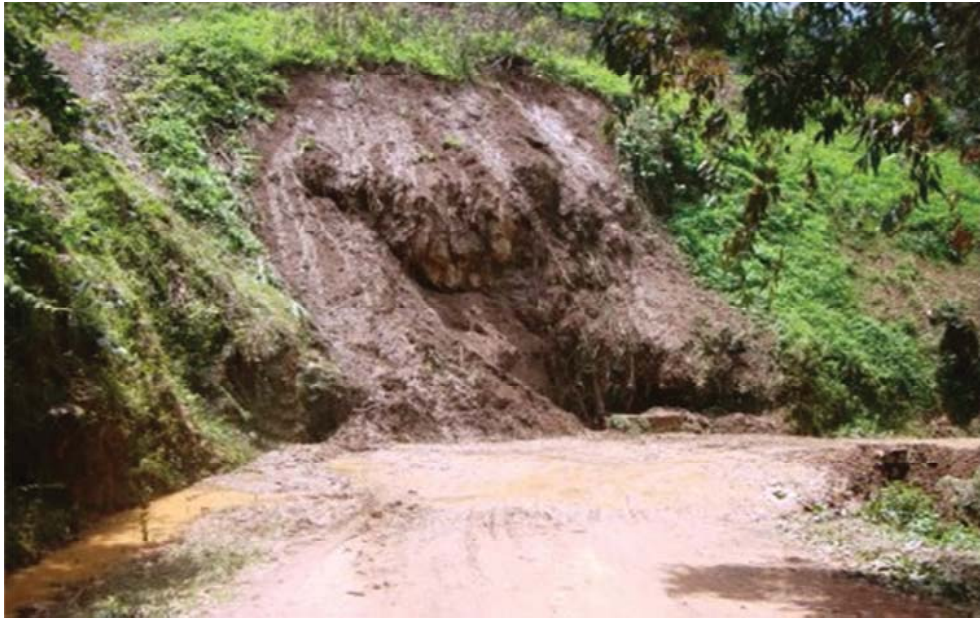
Figure 8. Land degraded in Rwamagana District due to floods in 2012
